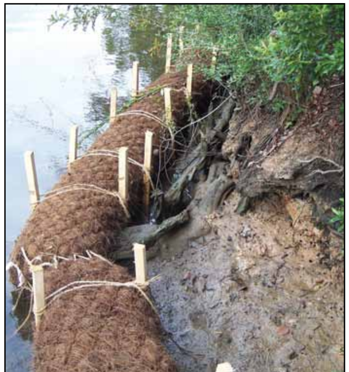
Coconut fiber logs placed along an eroding shoreline in the Gulf Hills Community of St. Martin.
